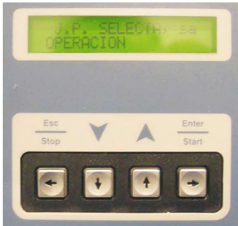
Fig 5.1 Panel de control.
