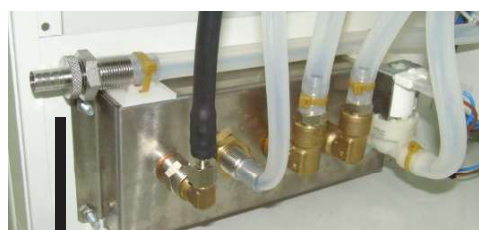
Cooling circuit valve
